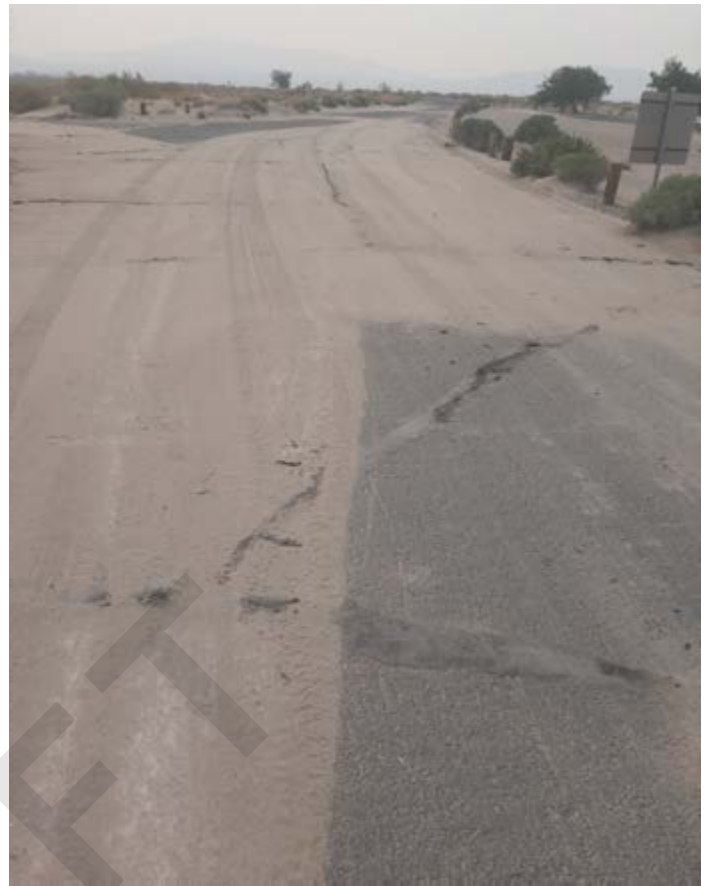
Sand accumulation on a road in the Lahontan Dam region
