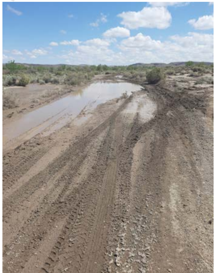
Water and use damage on a gravel road
