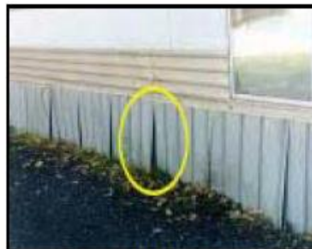
Fix gaps in trailer skirtings
