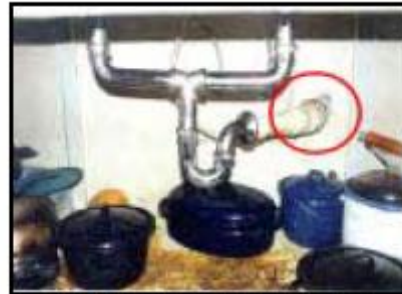
Look for gaps where the water pipes come into your home
