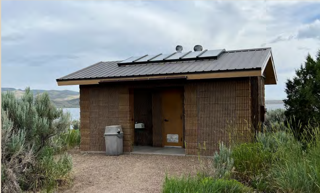
Exterior view of the Day-Use Restroom. Constructed in 1982, this facility is in dire need of replacement.
